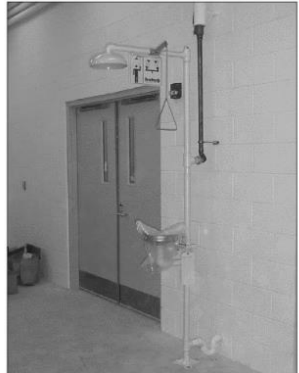
Commentary Figure 411.1 EMERGENCY SHOWER AND EYEWASH STATION (Photo courtesy of B&I Contractors, Inc.)
