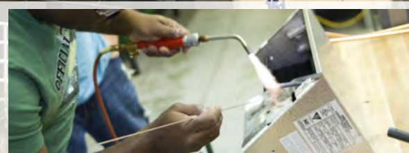
HVAC / Refrigeration Technology
